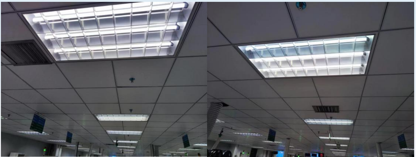
100% coverage of workshop LED lights
